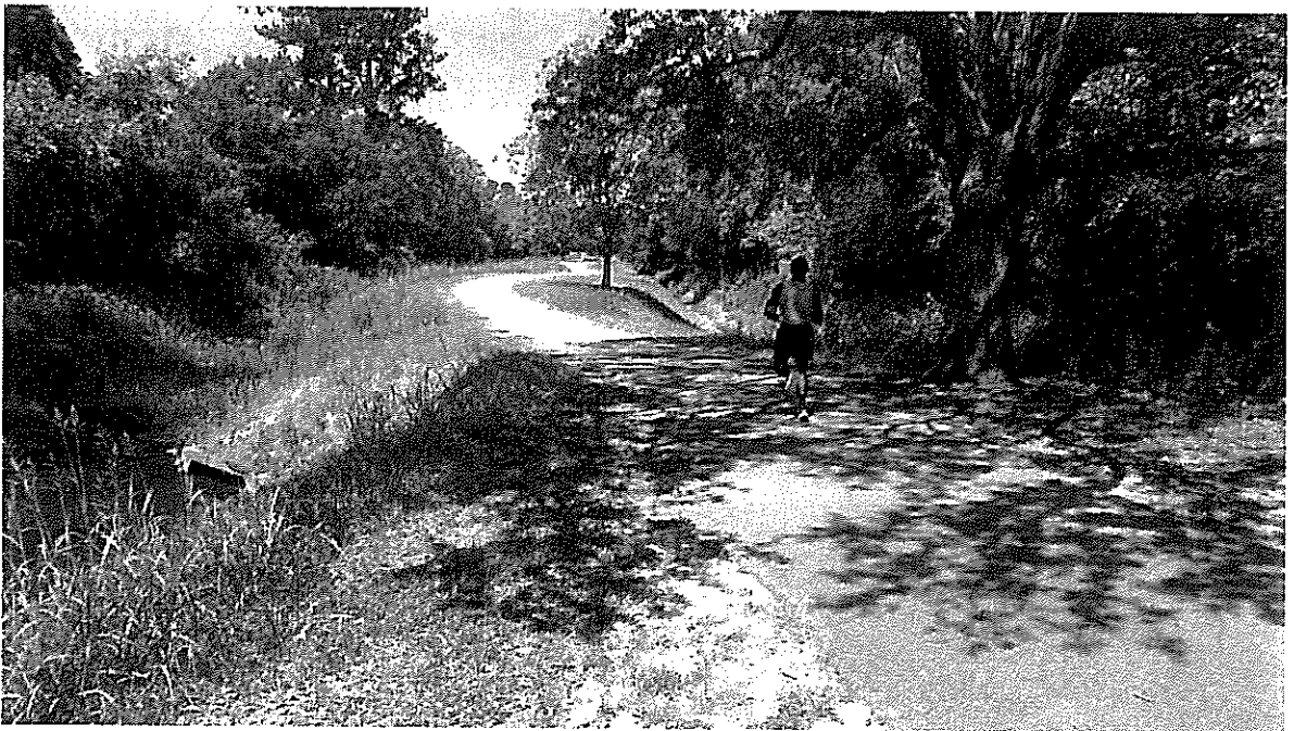
Ardmore culvert (view West). Widening the path will likely require Safety Barrier on both sides of the path in some areas. The existing shoulders are as narrow as 3' in many locations, and the drainage channels limit flexibility.
