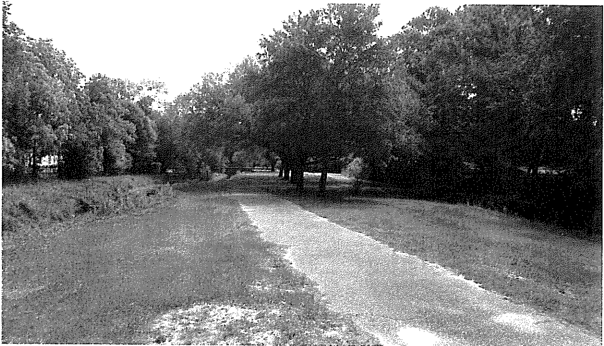
Approaching White Oak Drive (view East). The current path alignment has two bends winding through Live Oaks planted as part of the Ardmore project. Will seek to minimize disturbance in this area while addressing root damage and horizontal alignment issues.
