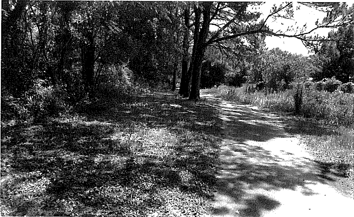
Nearing Wantoot Blvd. (view East). The pines ahead will have to be removed to correct the cross-slope and prevent future root damage.
