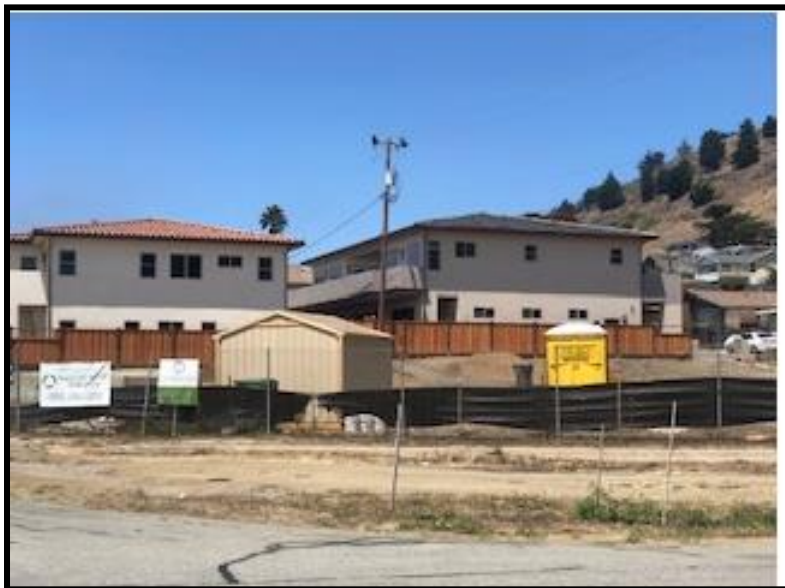
Recent construction on adjacent lots APN 064-263-053 and APN 064-263-025 - photo taken looking north-west
