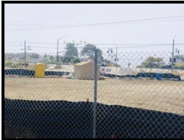
Looking west toward oceanfront from Orville Avenue after demolition of buildings, site is graded relatively flat
