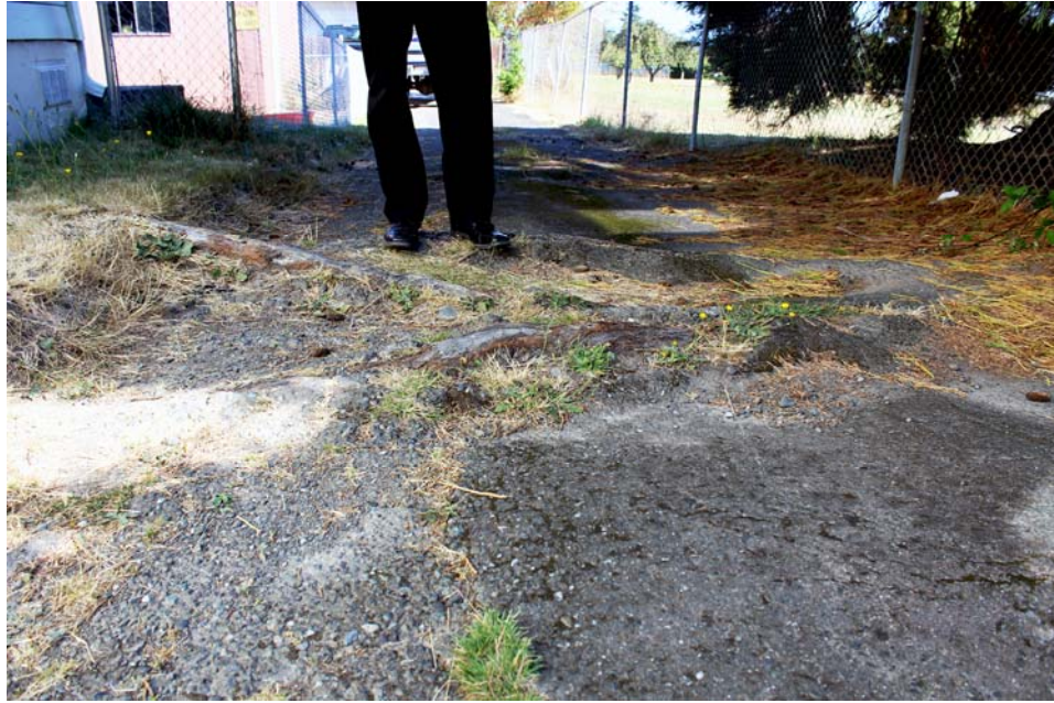
Photo 1 – Root Upheaval on Neighboring Property Driveway
