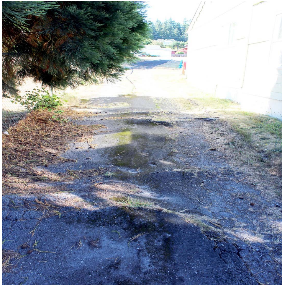
Photo 2 – Root Upheaval on Neighboring Property Driveway
