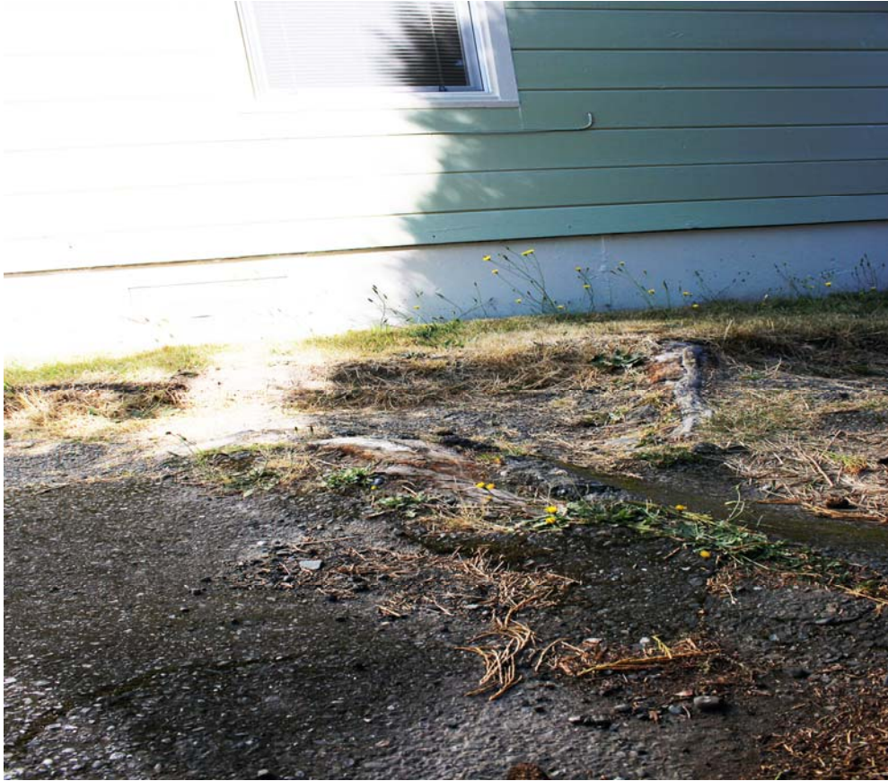
Photo 3 – Roots Under Neighboring Property Foundation
