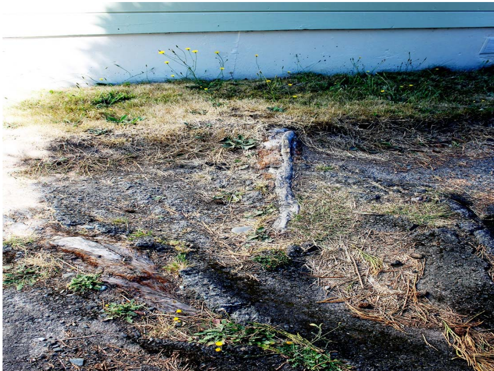
Photo 4 – Roots Under Neighboring Property Foundation
