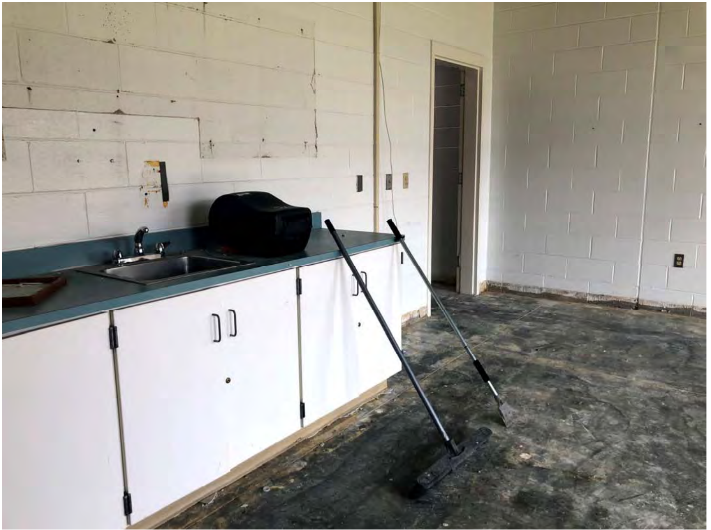
Existing Teacher Break Area: Some Flooring and wall mounted accessories removed. Flooring and Casework removal underway.
