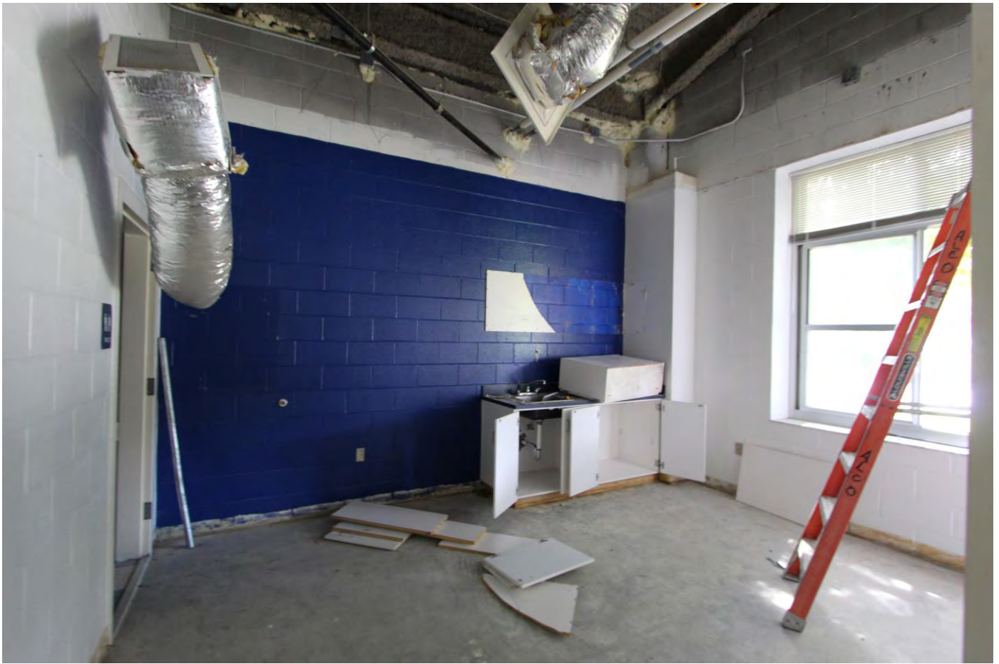
Health room A104, casework was not to be demo'ed, restroom door was not to be demo'ed
