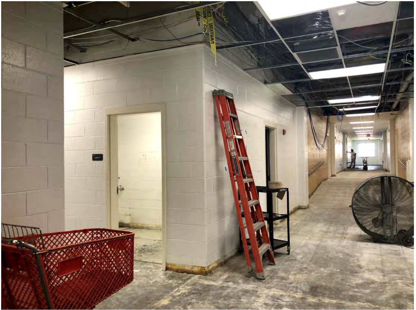
Existing Entry Hallway: Flooring, Ceiling Tiles, and some plumbing fixtures have been removed.
