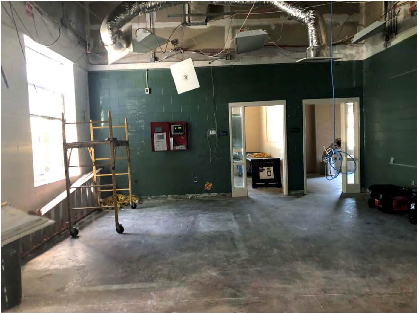
Existing Entry Lobby: Casework, some wall mounted fixtures, ceiling grid and tiles, and VCT flooring have been removed.
