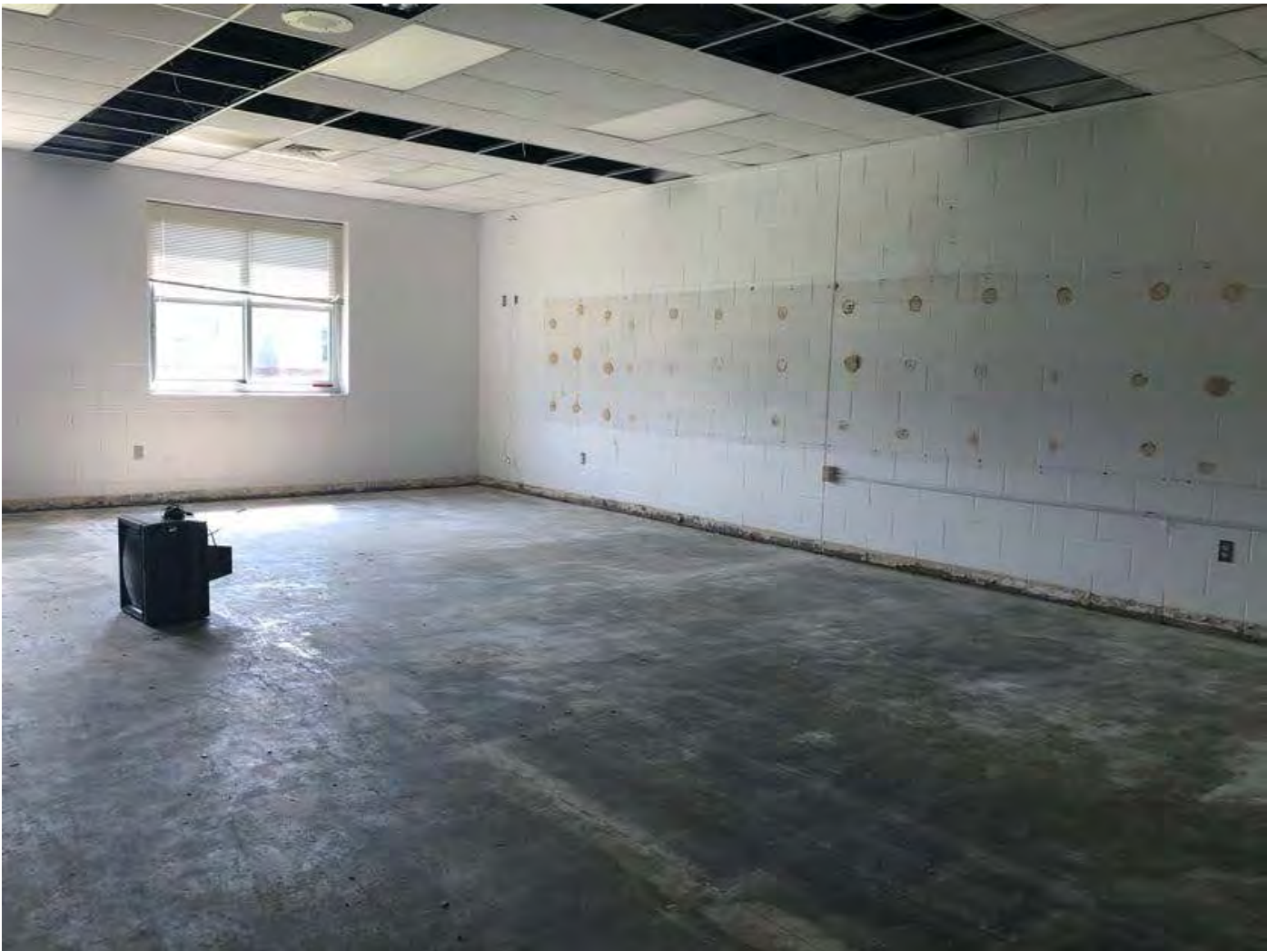
Existing Classroom Demo: Casework, flooring, base, wall mounted accessories, and ceiling tiles have been removed.
