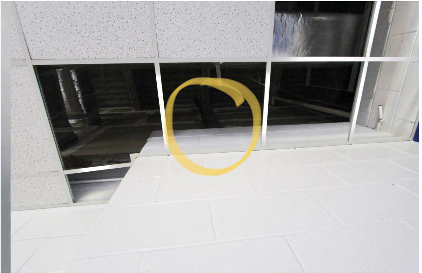
Classroom A120 bumpout is block not gyp, to be demoed and case around pipe
