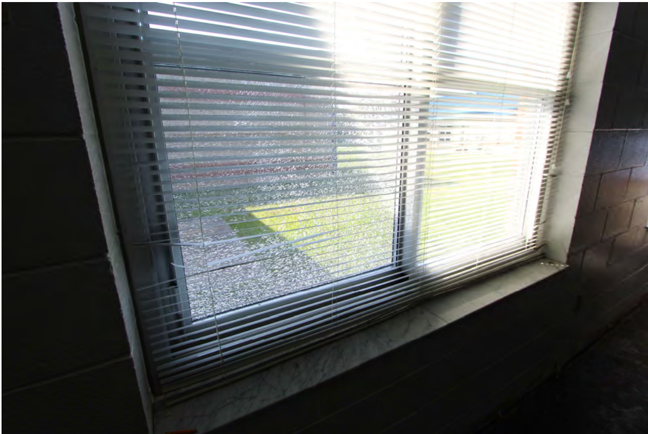
Broken window in room B132, outer pane of glass broken.
