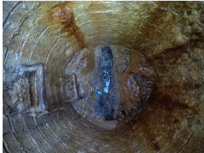
Manhole w/active infiltration (stains)
