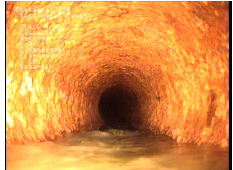
Cast Iron Pipe Severe Corrosion
