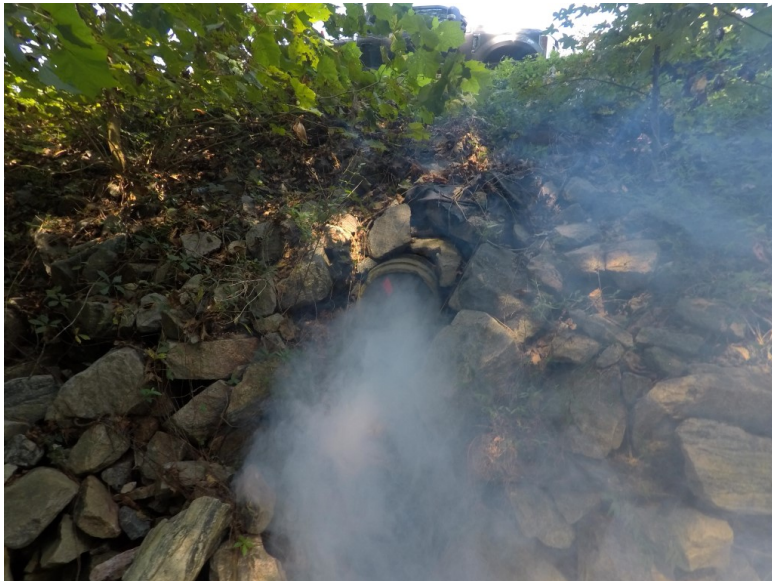
Storm Drain Cross Connection
