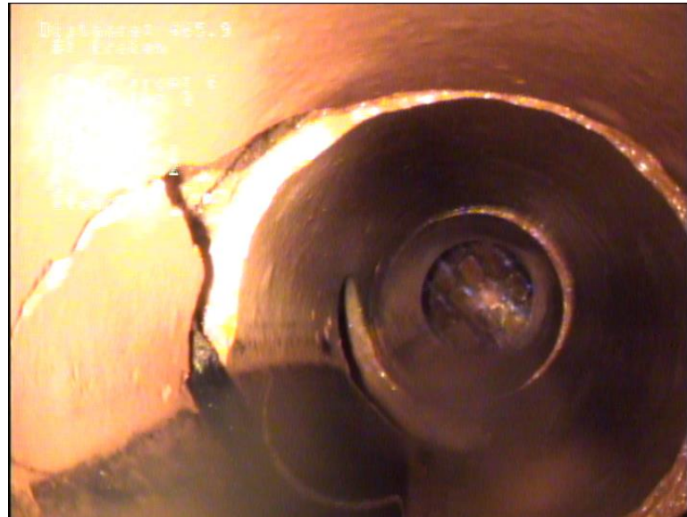
Severe Offset Joint w/Fracture
