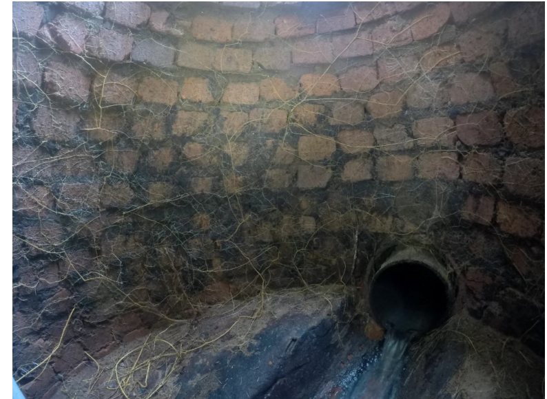
Root Intrusion in Manhole
