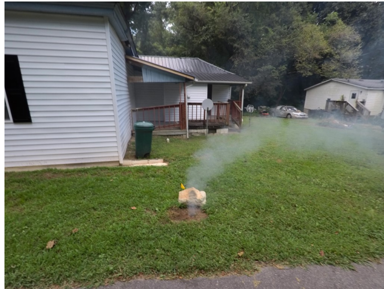
Leaking Clean-Out Cap
