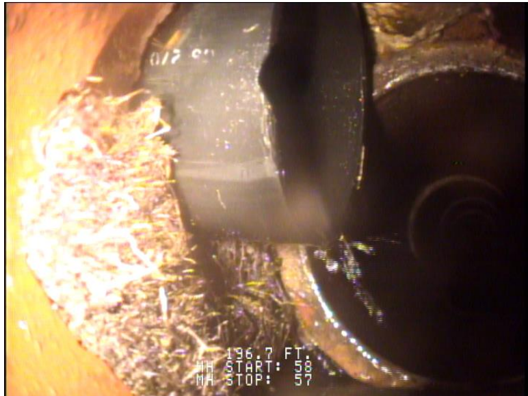
Protruding Hammer Tap
