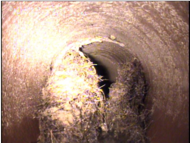
Severe Root Infiltration
