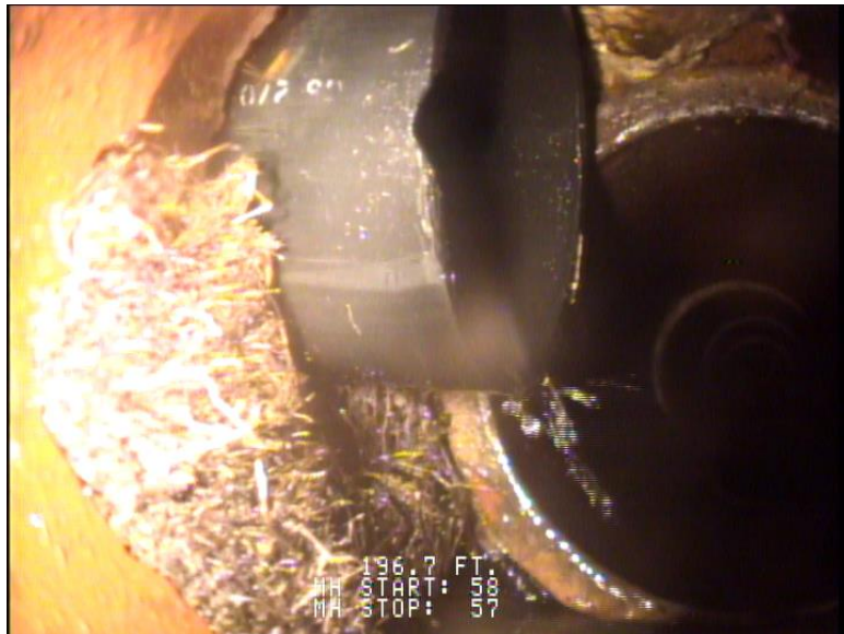
Protruding Hammer Tap
