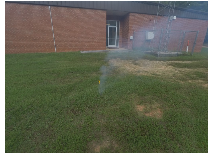
Defective Sewer Lateral
