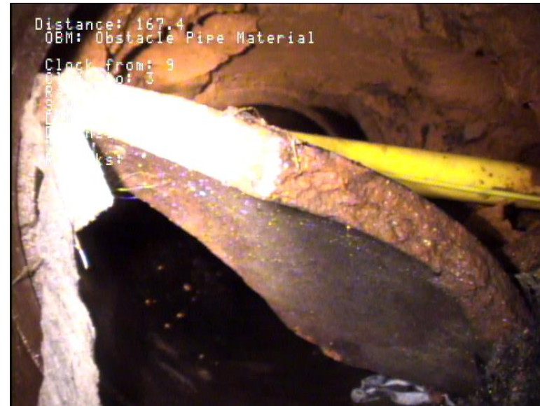
Gas Line installed through Sewer Pipe
