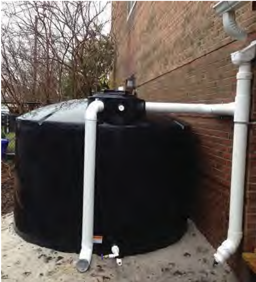
Figure 4.23. Example cistern application (photo: Marty Morganello).
